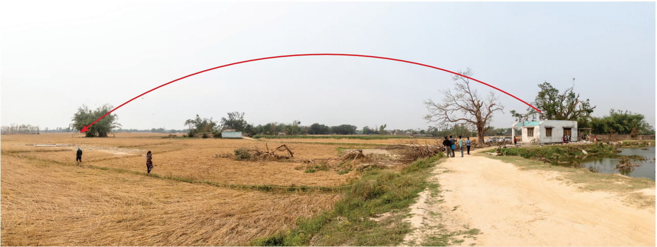
Figure 3.10b: Concrete roof of approx. 20 × 20 feet one story building blown away 80 m downstream (Gamhariya)
