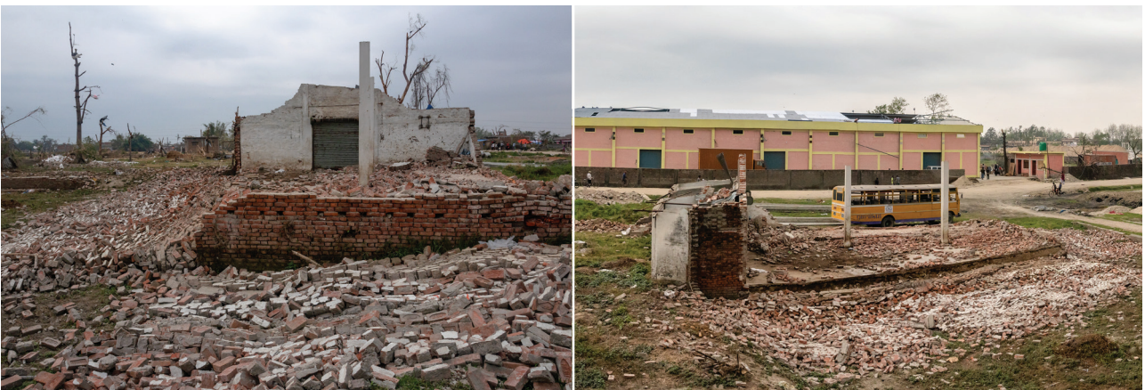
Figure 3.10d: Storage building: exterior brick walls with tin roof on metal frame collapse completely in Chainpur
