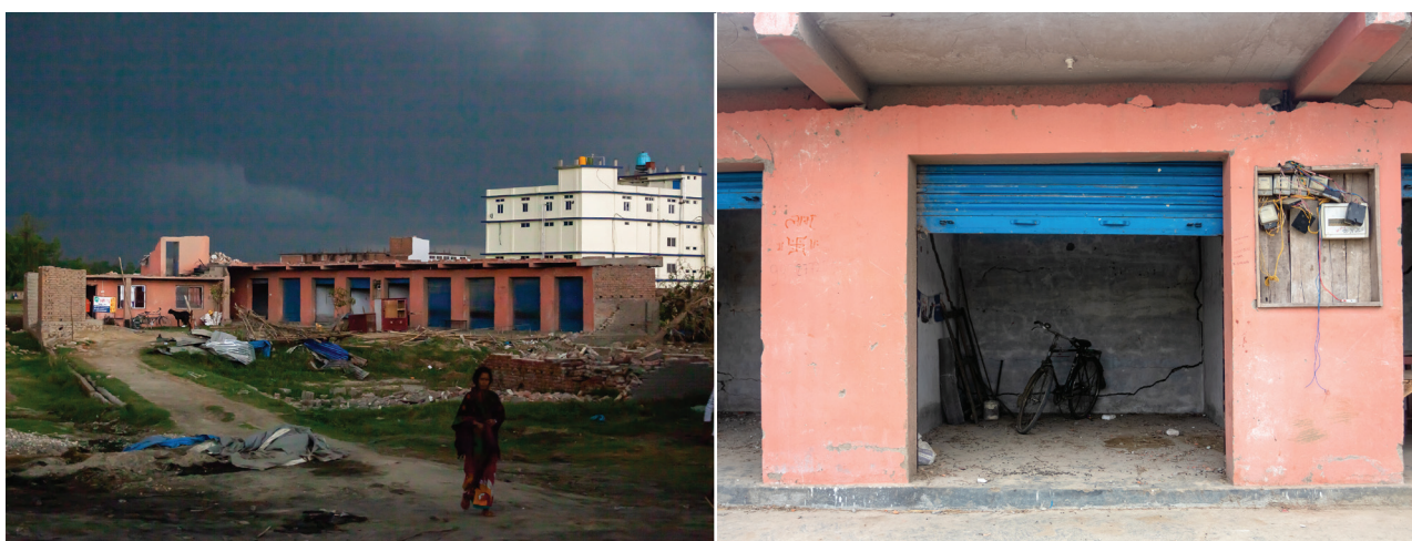
Figure 3.10a: Concrete roof of 100 × 12 feet, one-story building uplifted partially (Chainpur)
